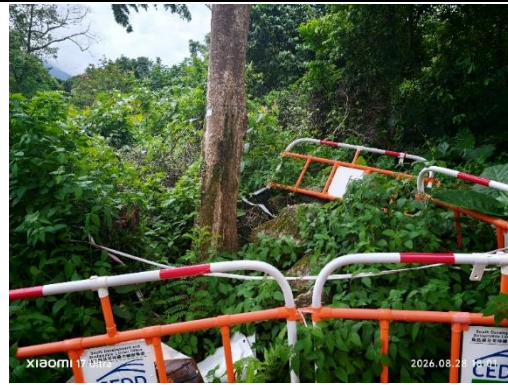
Photo 2. Tree C11-T0120: Tree base and fence
