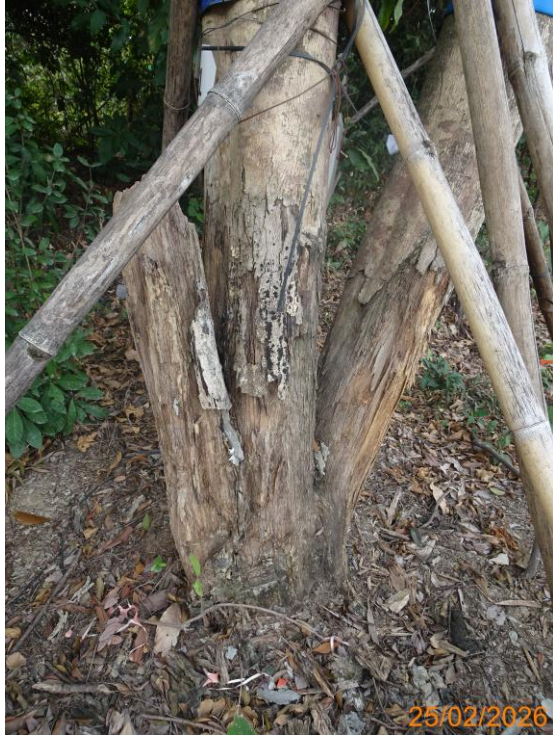
13: U041_ Wood damage at trunk union#1
