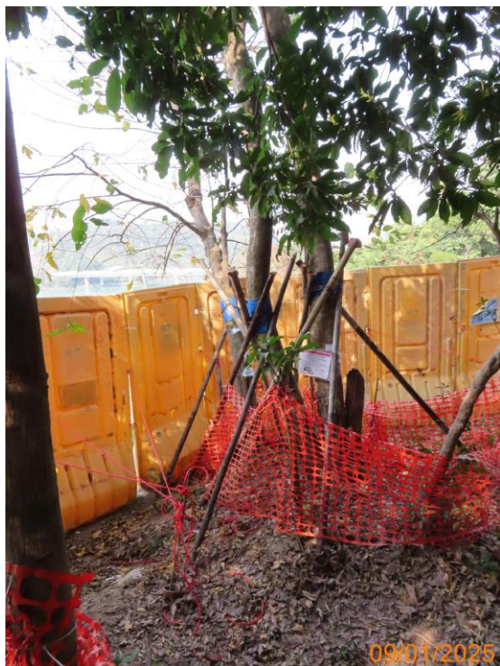
21: Temporary protective fencing for U041, U042 and U043
