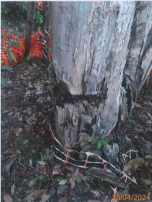
11: U041_Wood damage by termite
