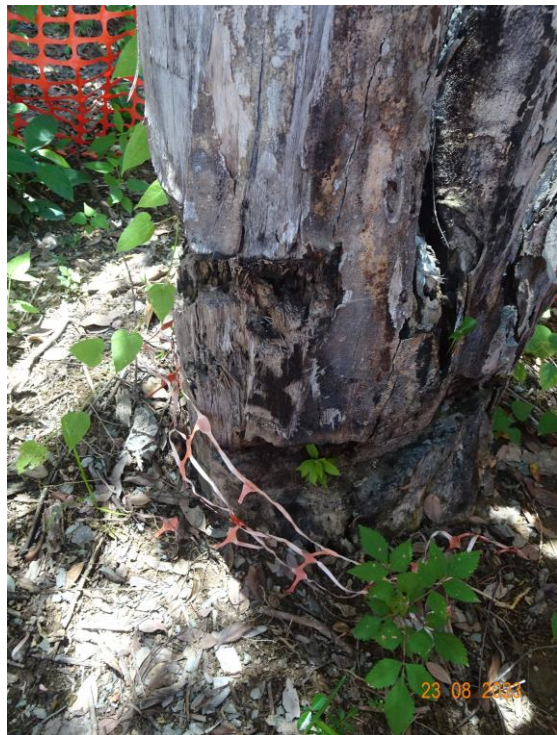
8: U041_Wood damaged by termite
