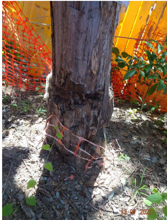
8: U041_Wood damaged by termite
