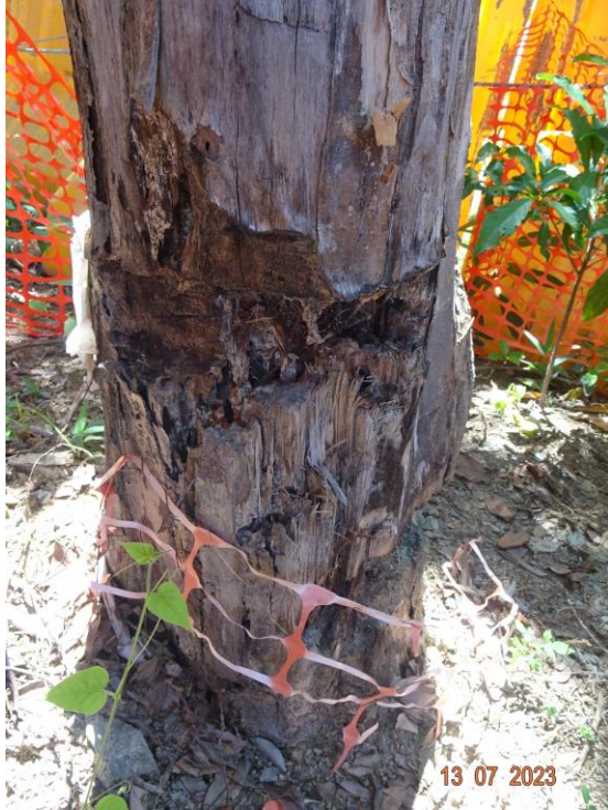
9: U041_Wood damaged by termite_Close up
