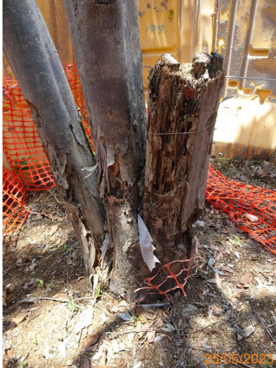
9: U041_Wood damaged by termite
