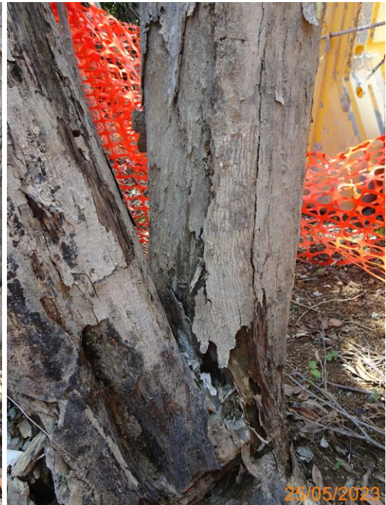
8: U041_Wood damage at union
