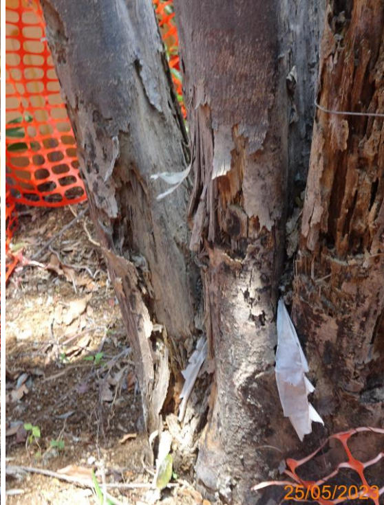
10: U041_Wood damaged by termite (Close up)
